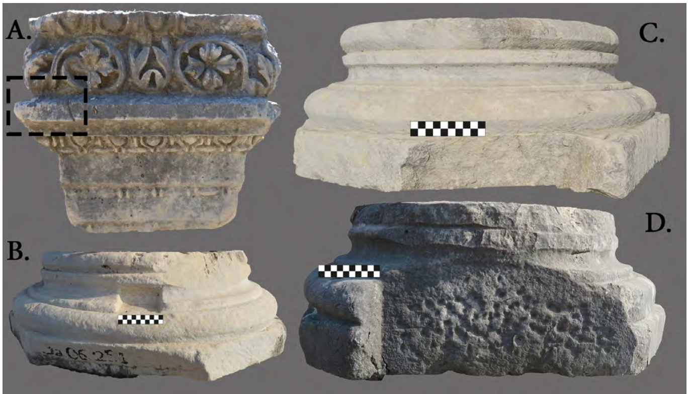
Fig. 9a-e. Examples of Type C repairs at Perge. A: Architrave of the palaestra of the South Bath-Gymnasium. B-D: Repairs on the attic-ion type pedestals on the colonnaded street running north-south.
